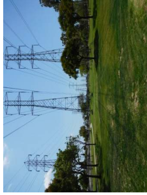
2. Looking South on SCE Corridor
