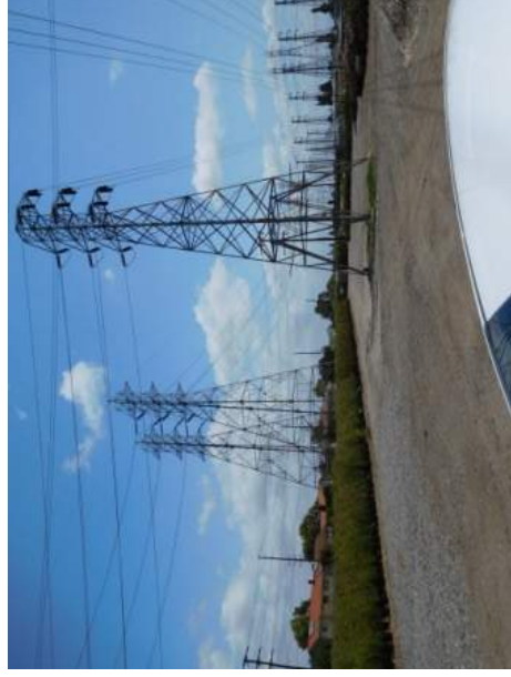
2. At SCE Transfer Station looking East
