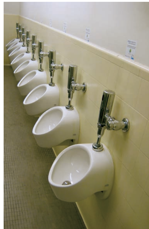
Installation of low-flow urinals in bathrooms on the University of California at Los Angeles campus is one of many Metropolitan-assisted projects in the Public Sector Program which demonstrates leadership in water-use efficiency by public agencies.
