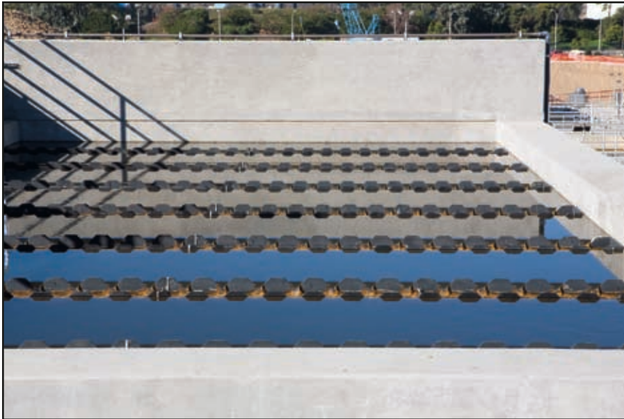
The West Basin Water Recycling Facility is one of the largest recycling plants in the nation located in El Segundo, California.
