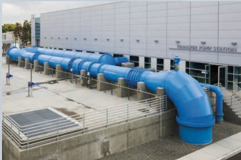
Orange County Water District's Groundwater Replenishment System treats up to 75,000 acre-feet of wastewater for groundwater recharge.
