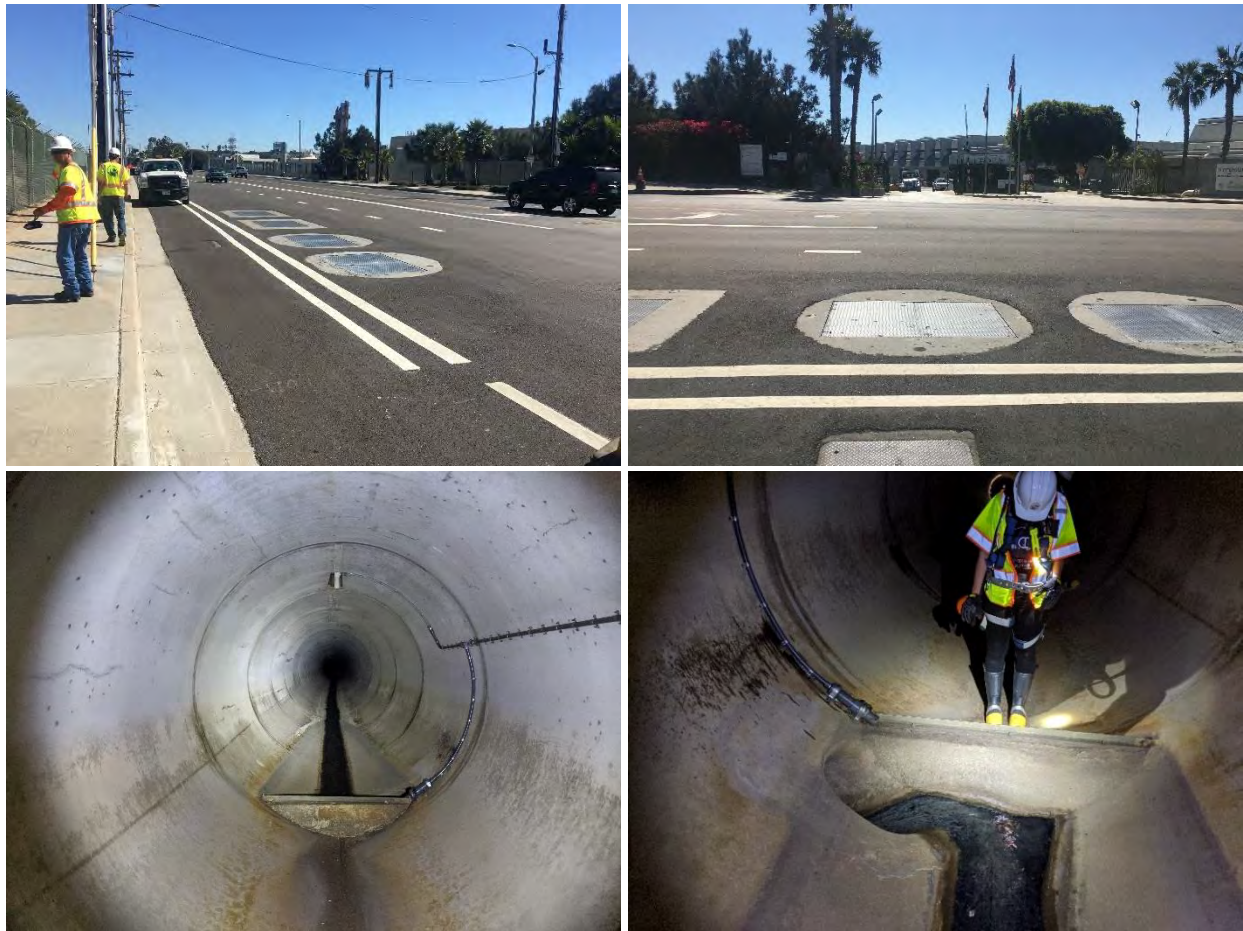
Photo 4-4. Pershing Drive DWD; Photographs Taken during the October 22, 2019 Site Visit with Los Angeles County Flood Control District Staff
