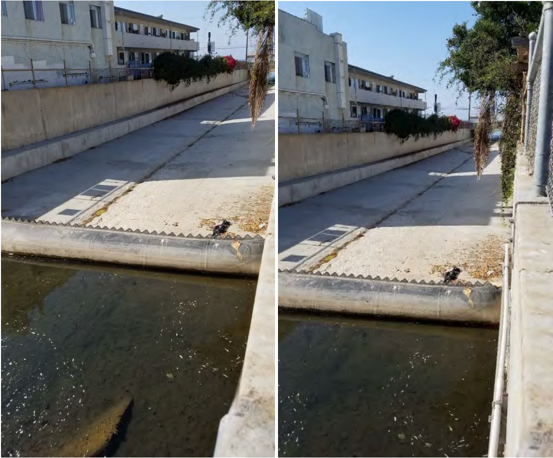
Photo 6-2. Example Diversion Structure with an Inflated Rubber Dam Photograph Taken during the October 15, 2019 Site Visit with Los Angeles Sanitation and Environment Staff
